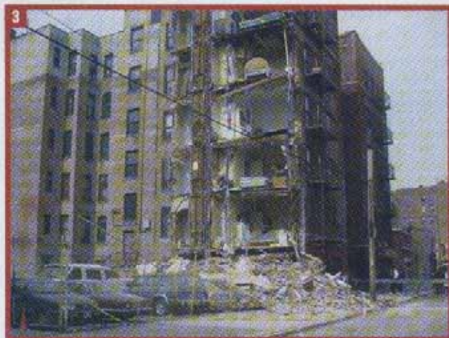
(3) At this type of building collapse, expect damaged interior gas pipes and suspect damaged in-ground pipes. Have the utility shut the gas to the building and check for leaks in the street.
