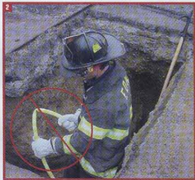
(2) A firefighter easily bends this plastic pipe, but doing so could result in a static spark that ignites leaking gas. Do not approach or touch leaking plastic pipe.
