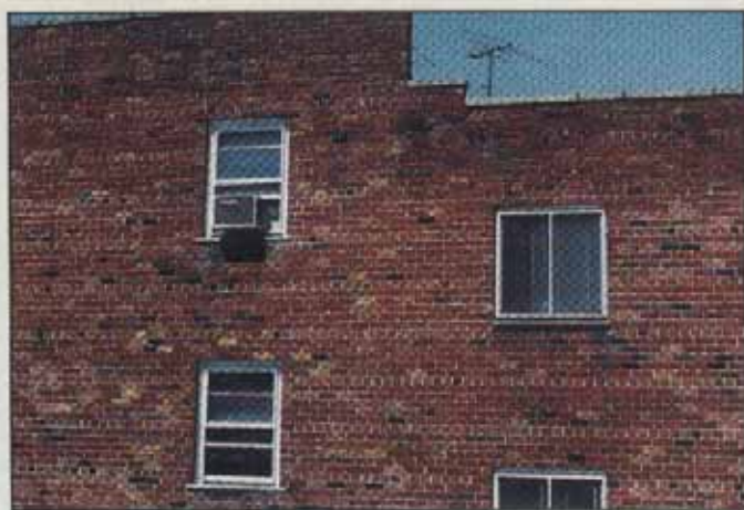
The staggered window placement at the side of a building may indicate a split-level configuration.
